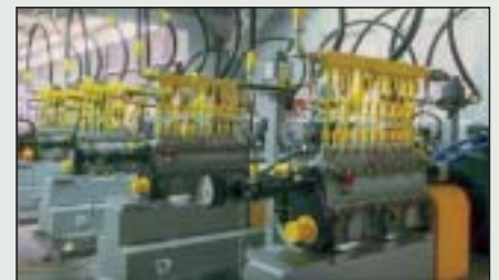
Multi-component metering group with high efficiency pumps.
